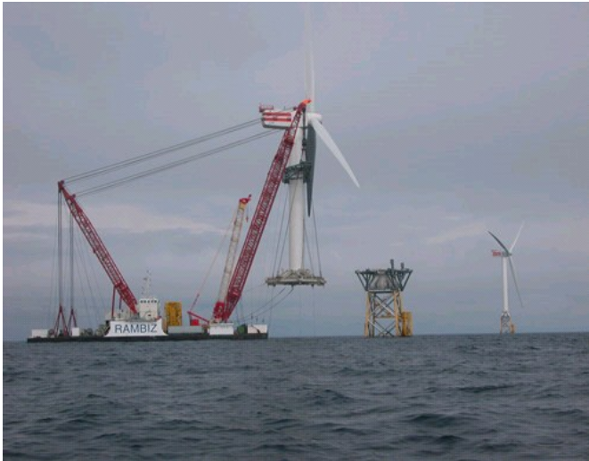
Figure O: Photograph of a heavy lift barge installing an offshore wind turbine. (Source: Saldis Salvage and Marine Contractors)
